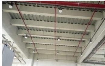
Sprinkler system at warehouse
