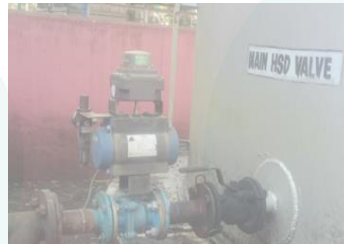
Auto Shut off Valves
