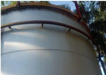
HSD tank cooling System
