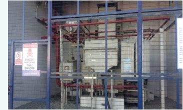
Sprinkler system at transformer yard
