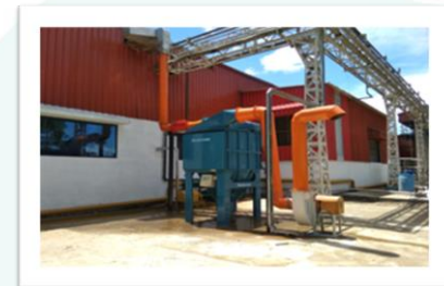
Dust Collector for elimination of dust
