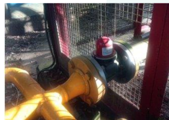
Seismic Shut off Valve
