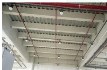
Sprinkler system at warehouse
