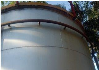
HSD tank cooling System
