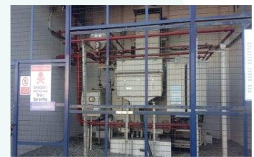
Sprinkler system at transformer yard
